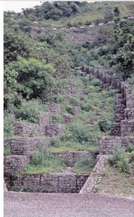
c) Continuous gabion cascade protecting central drainage line from scour
