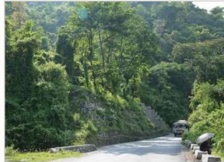
a) Gabion retaining walls to support unstable slopes
