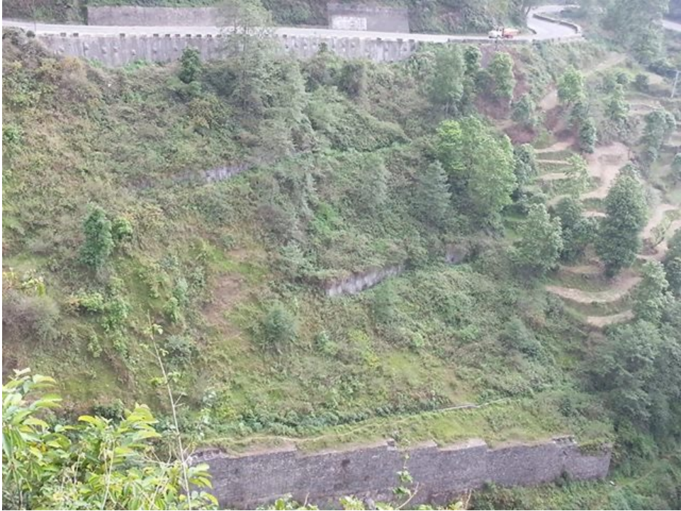
Khatripauwa Landslide TN10A
