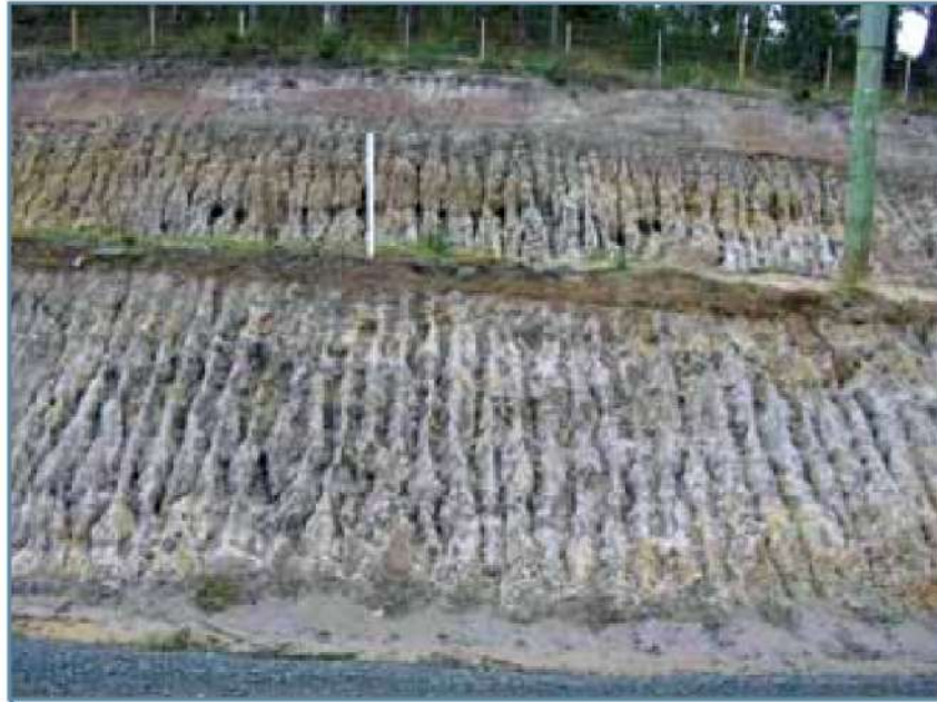
Figure 28. Rill and tunnel erosion caused by excavation of sodic soils for road construction. Dunalley.
